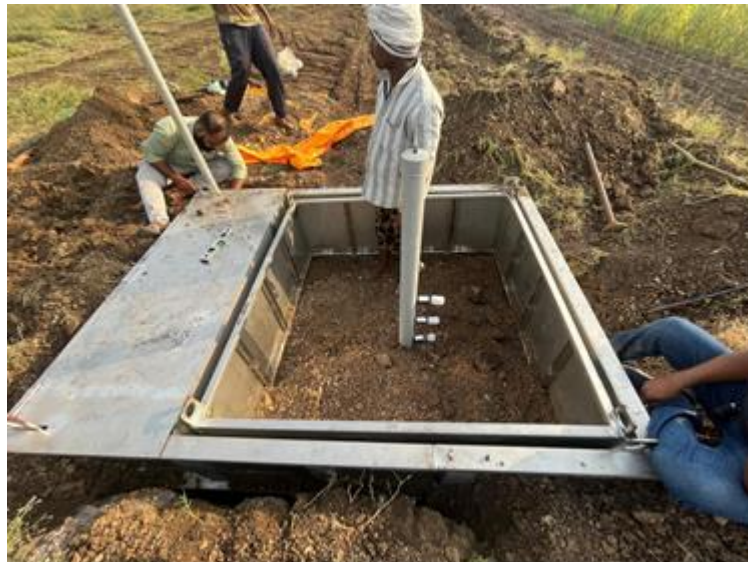
Plate 8. Layer wise soil refilling & compaction and sensor installation in the inner tank of Lysimeter
